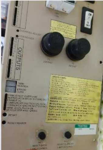
912C0137-06 Tank Control I/O Block
